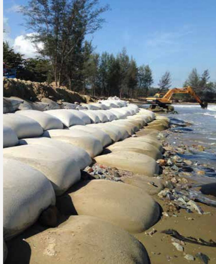
Bontec SNW Many sandy beaches around the world are subjected to ongoing erosion. Locally filled geobags can protect these beaches and the nearby infrastructure.
